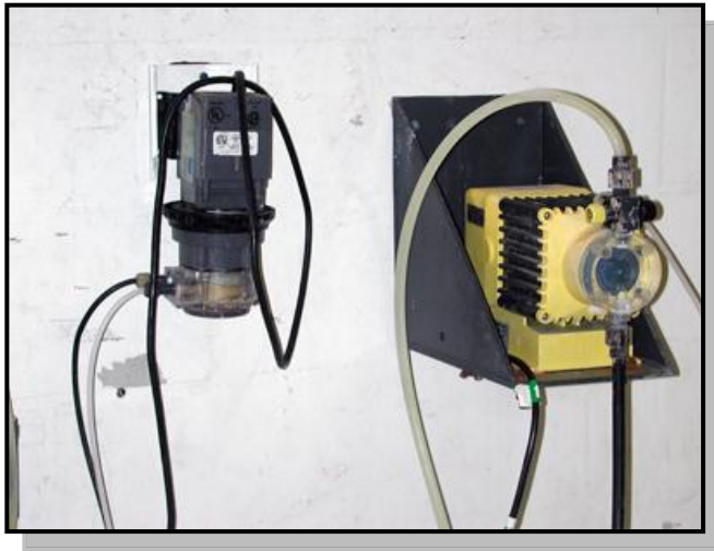
Liquid Chlorine and Acid Feeders
