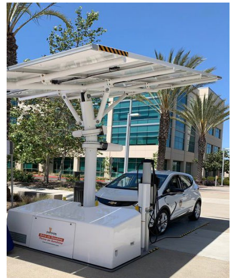
Exhibit 2-3: PV to EV Unit at COC
