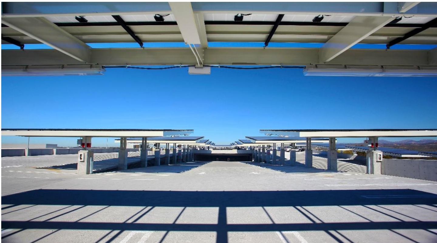
Image: PV system located at COC Parking Structure A
