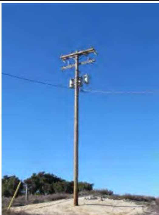
Photograph 20. Pole mounted transformer on the Lansing property.
