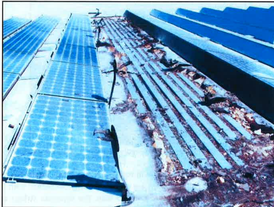
Figure 2-12: Fire-Damaged Array in April 2009 CA Incident 46
