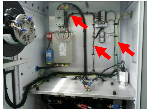
Controlled Wire Routing
