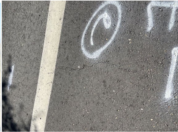
Photo 2-3-4: Skyline TT 18 Months. Representative hairline cracking
