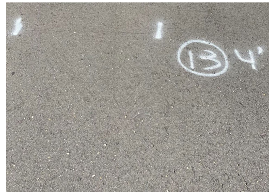
Photo 2-2-4; Skyline TT 18 Months- closeup of hairline cracking
