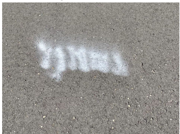
Photo 2-4-4: Skyline TT 18 Months Close up of Hairline cracking
