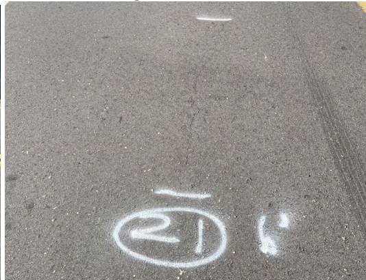
Photo 2-1-4; Skyline TT 18 Months- closeup of hairline cracking
