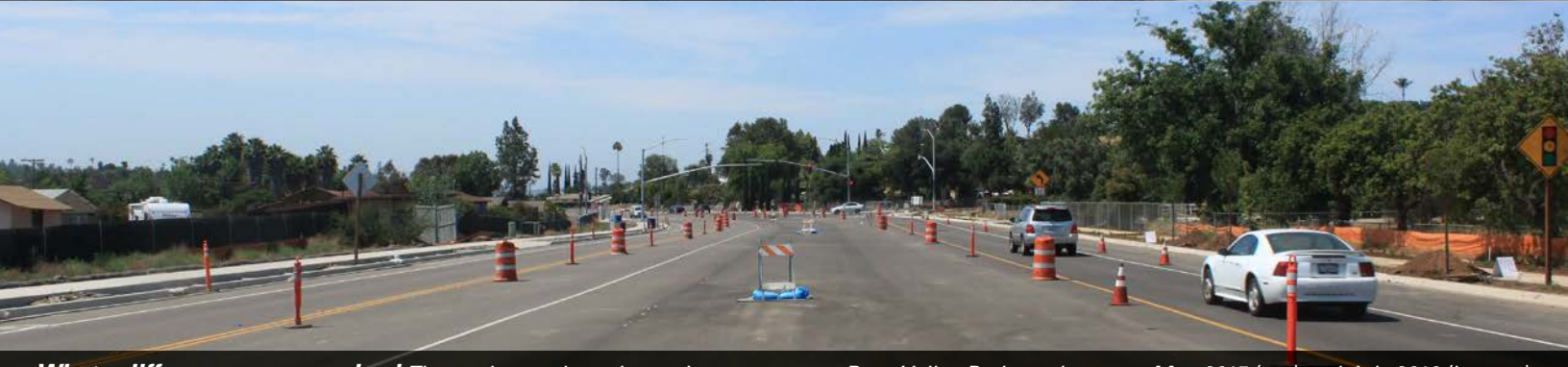
What a difference a year makes! These photos show the paving progress on Bear Valley Parkway between May 2015 (top) and July 2016 (bottom).
