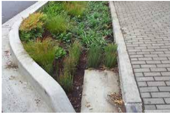
Permeable pavement sidewalk with biofiltration
