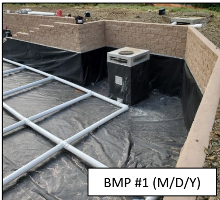
Sub-surface liner, underdrain, and outlet structure
