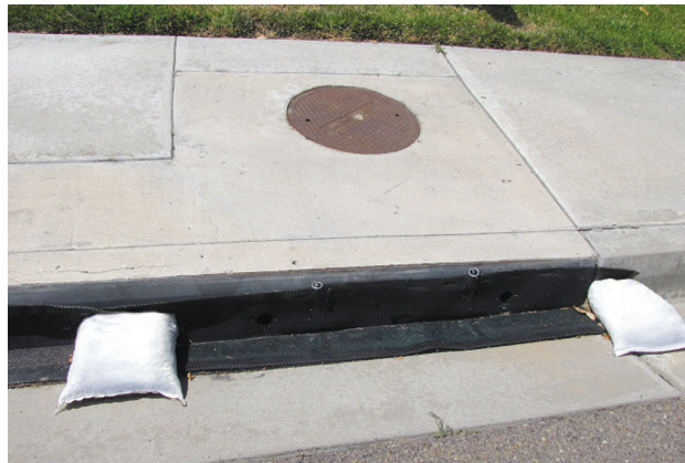
May takip na storm drain
