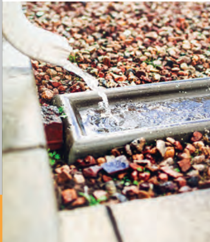
Downspout and splash block
