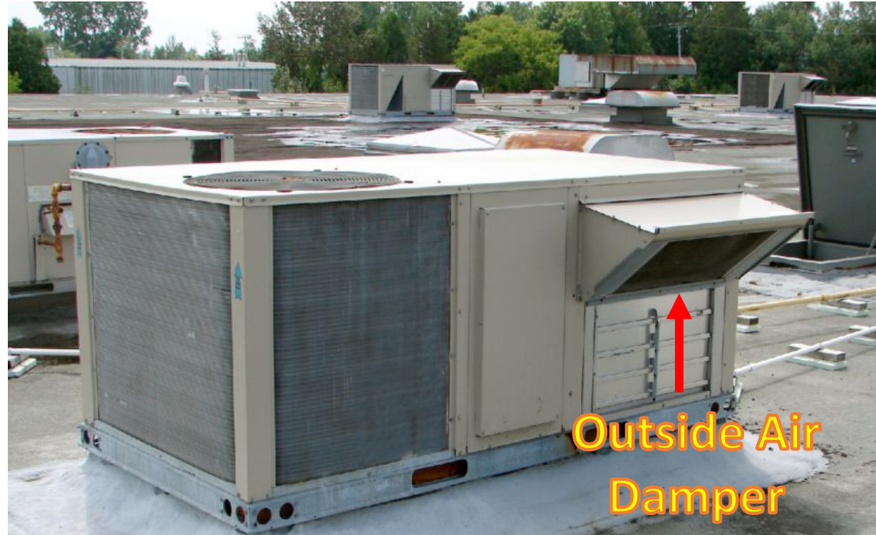
Adjustable Ventilation Damper
