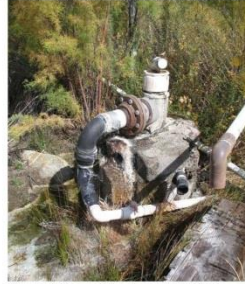
Figure 4 One well in close proximity to Jacumba Lake is under pressure and the upwelling water is currently filling the historical splash ponds with several feet of water. This water could be used to refill and maintain Jacumba Lake.
