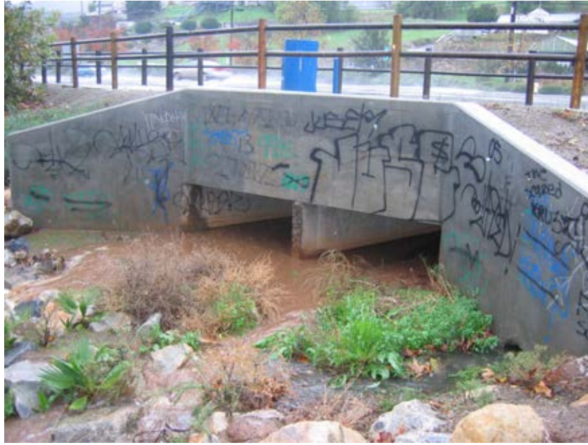
Basin 1 Outlet- East Side Twin Oaks Valley Road
