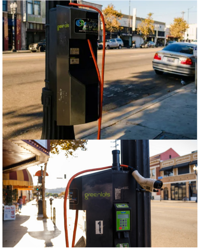
Examples of on-street EV infrastructure
