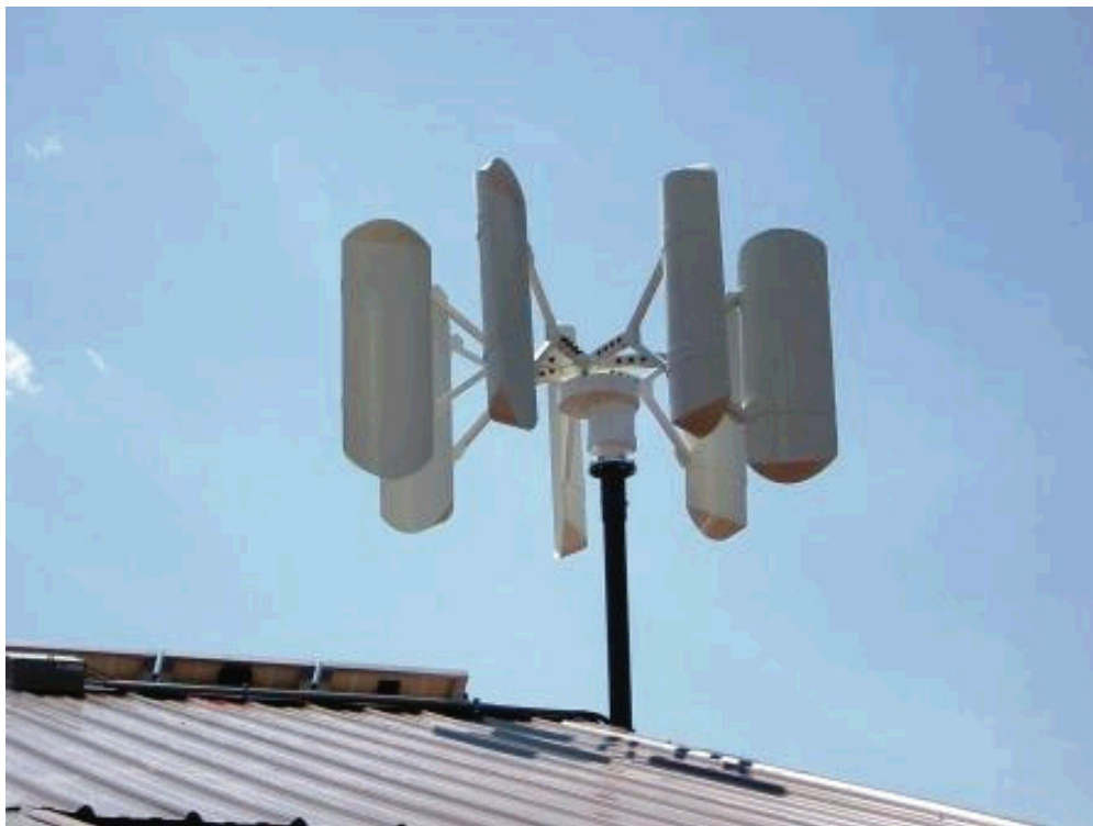
Roof Mounted Vertical Axis Turbine
