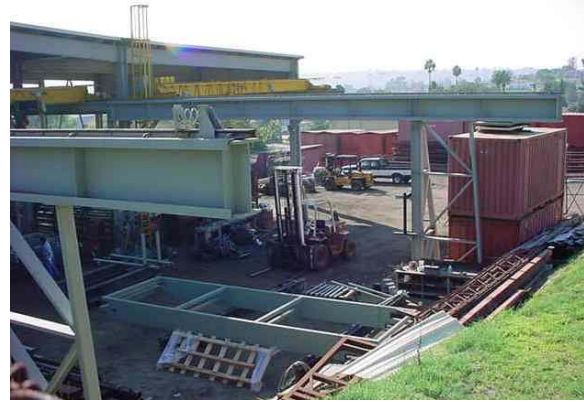
Steel fabricating plant in Spring Valley
