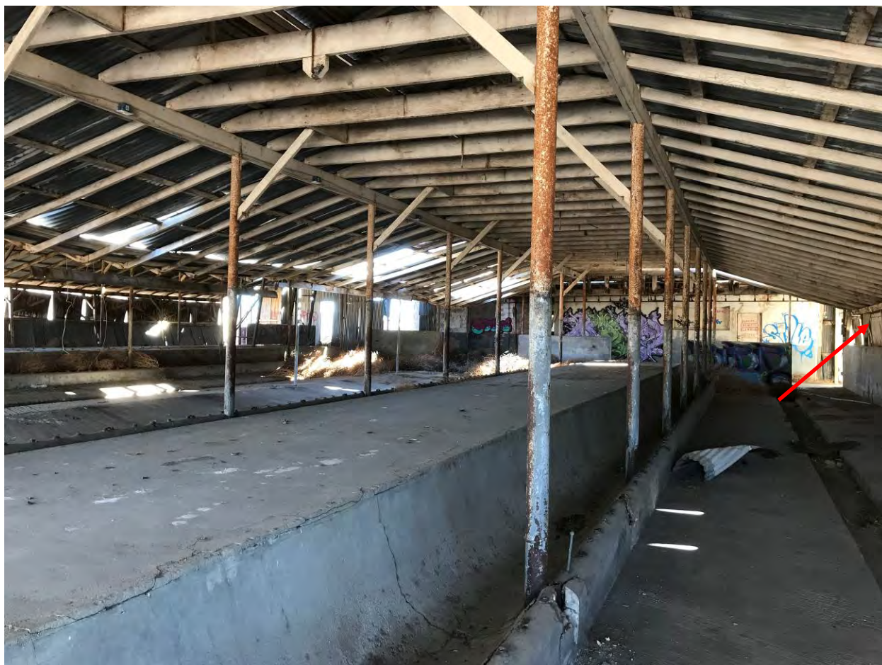
Photo 22 – Ground level view of the inside of room 6 in Building 4D. The wall framing on side D (red arrow) and metal posts throughout the center of the room were all found to contain elevated lead levels.
