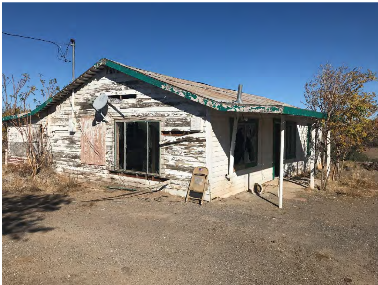
Photo 16 – Ground level view of the north and east sides of Building 2. The window frames, eaves, and wood siding on all four sides of the building were all found to contain elevated lead levels. Photo not included of hall opening on side D and door and door frame on side A in living room; window on side D in kitchen; window, window frame, and window sill on side B in porch; closet door on side C in hall; and door on side B in restroom; window frame on side A in bedroom 1 on inside building 2 that were also found to contain elevated lead levels. Joint compound was found to contain asbestos, however composite of wall system (drywall, joint compound, off-white compound and drywall tape) located throughout the building was found to contain less than 1% of asbestos .
