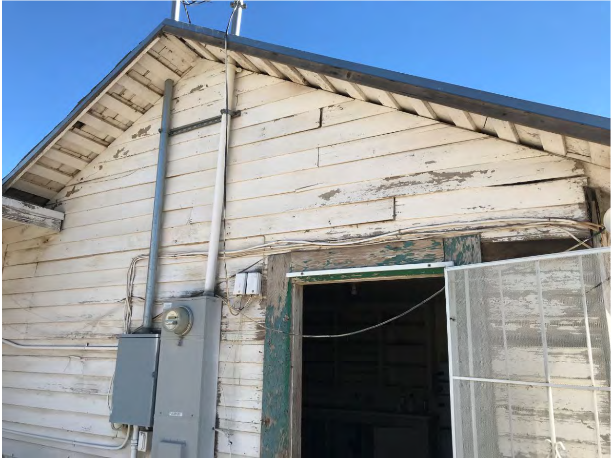
Photo Five – Close up photo of wood siding and eaves on exterior of building 5 that were found to contain elevated lead levels.
