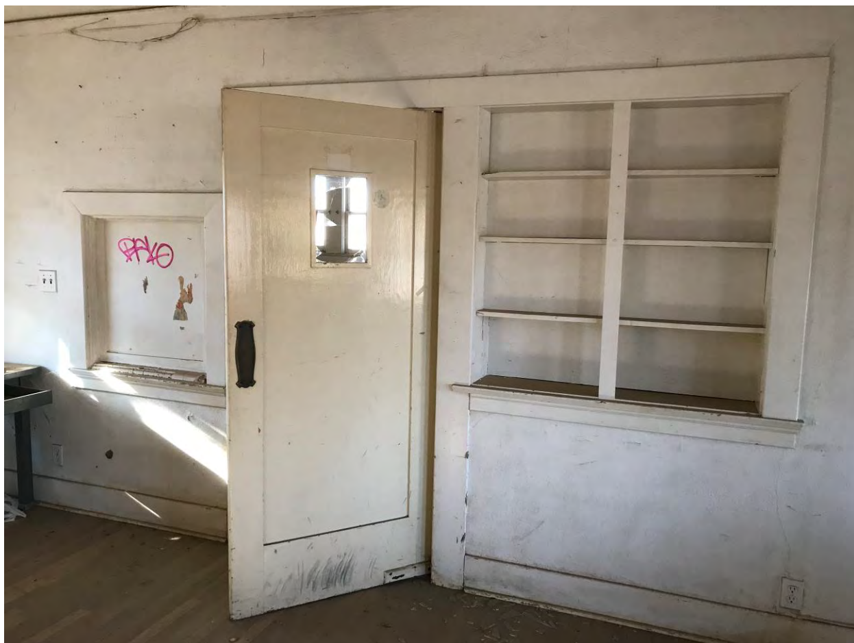
Photo 10 – Photo of access window, shelves, baseboard, door, and door frame on side A of dining room in building 6 that were found to contain elevated lead levels.
