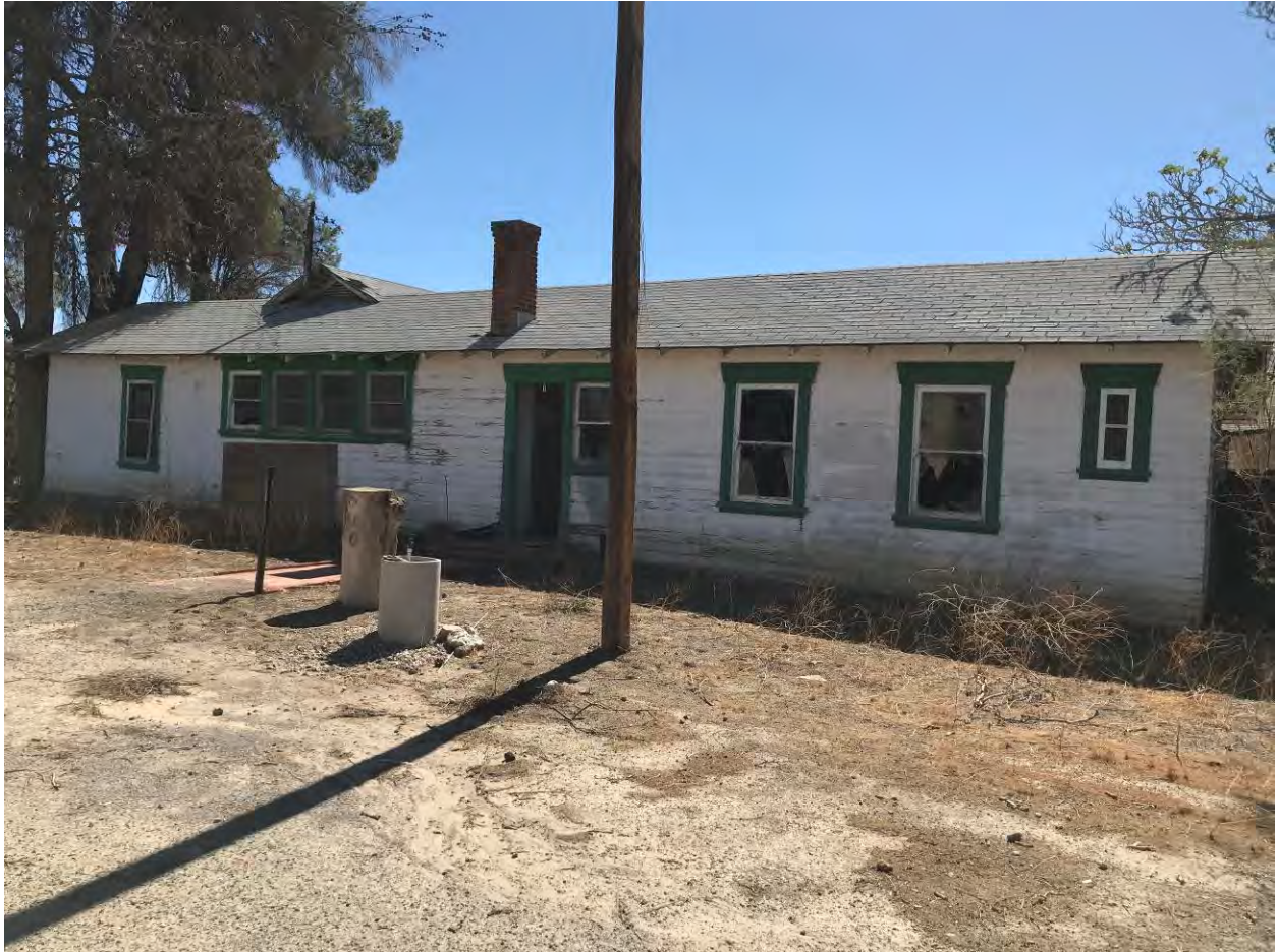
Photo Seven – Ground level view of the north side of Building 6. The windows, window frames, window sills, doors, door frames, wood siding, eaves, fascia, trim, and vents on exterior of the building were all found to contain elevated lead levels. Photos not included of upper shelves on sides B and C of living room closet and lower portions of walls covered with wallpaper in south hallway closet inside building 6 that were also found to contain elevated lead levels.
