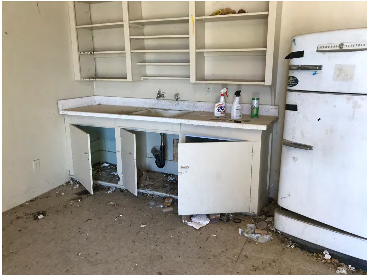
Photo Six – Photo of porcelain sink on side B of kitchen in building 5 that was found to contain elevated lead levels. The joint compound located throughout the building was found to contain asbestos.
