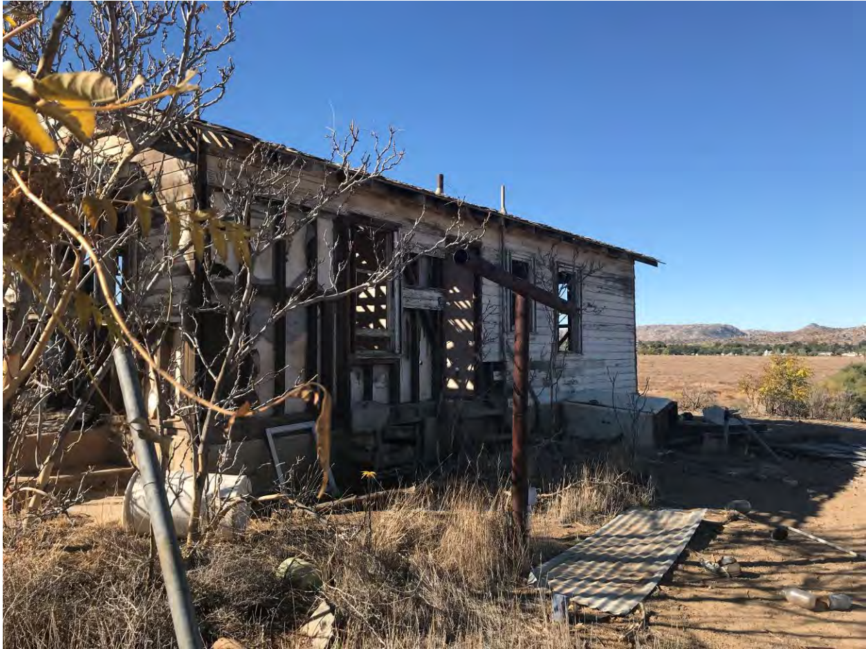
Photo 17 – Ground level view of the east side of Building 1. The windows, window frames, door frames, and wood siding on all four sides of the building were all found to contain elevated lead levels. Photo not included of windows, window frames, doors and door frames in laundry room and door on side B and window frame on side A in bedroom 2 on inside building 1 that were also found to contain elevated lead levels. The window putty located on the exterior of the building was found to contain asbestos. Joint compound was found to contain asbestos, however composite of wall system (drywall, joint compound, off-white compound and drywall tape) located throughout the building was found to contain less than 1% of asbestos.
