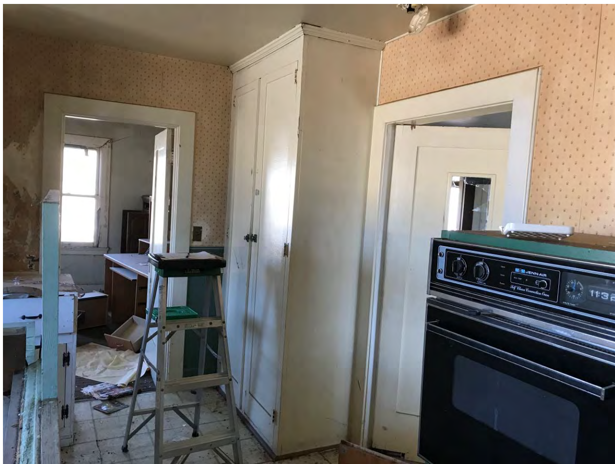
Photo Nine – Photo of pantry walls on side C, and doors, and door frames on sides B and C of kitchen in building 6 that were found to contain elevated lead levels.
