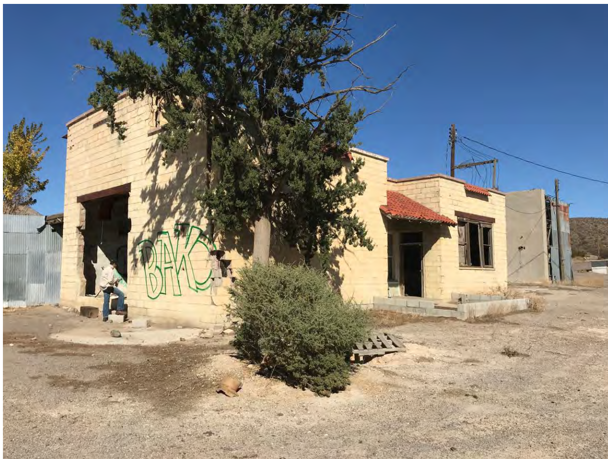
Photo 20 – Ground level view of the south and west sides of Building 4C. The windows, window frames, door frames, eaves, and eave beams on all four sides of the building were all found to contain elevated lead levels. Photo not included of concrete walls on all 4 sides, and door frame on side D, and window and window frame on side C in room 1; concrete wall on side B, door frame on side D, windows, window frames on side C, and stucco ceiling in room 3; plaster walls on all 4 sides, and door frame on side B in room 4; windows in chemical storage room; and window frames steps to overlook on inside of building 4C that were also found to contain elevated lead levels.
