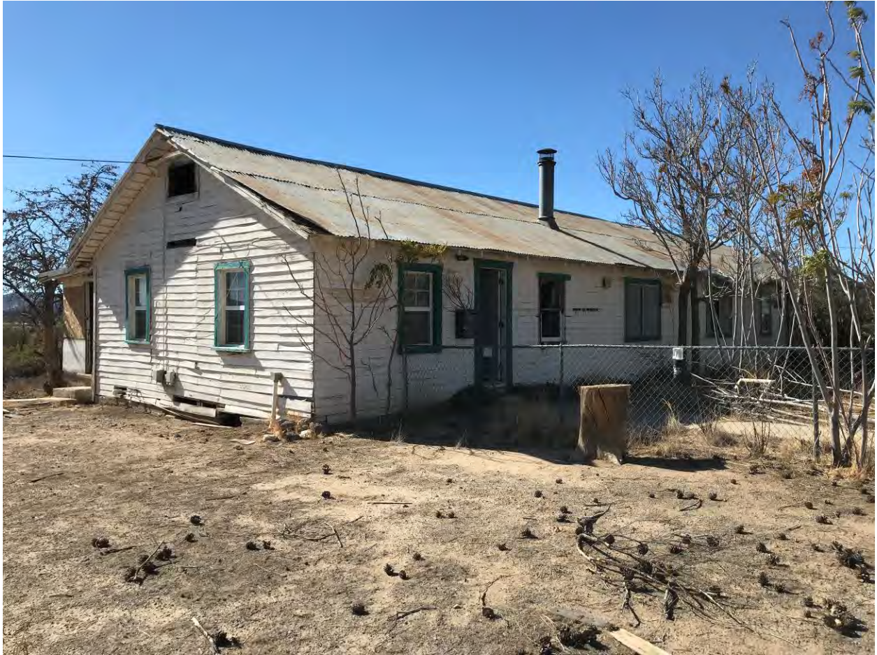
Photo 15 – Ground level view of the north and east sides of Building 7. The old windows on side A, and wood siding and eaves on all four sides of the building were all found to contain elevated lead levels. Photos not included of door frame on side A of east porch and door on side A of west restroom inside building 7 that were also found to contain elevated lead levels.
