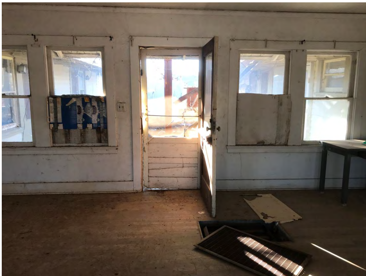
Photo 11 – Photo of windows, window frames, window sills, crown molding, baseboard, screen door, and door frame on side B of dining room in building 6 that were found to contain elevated lead levels.
