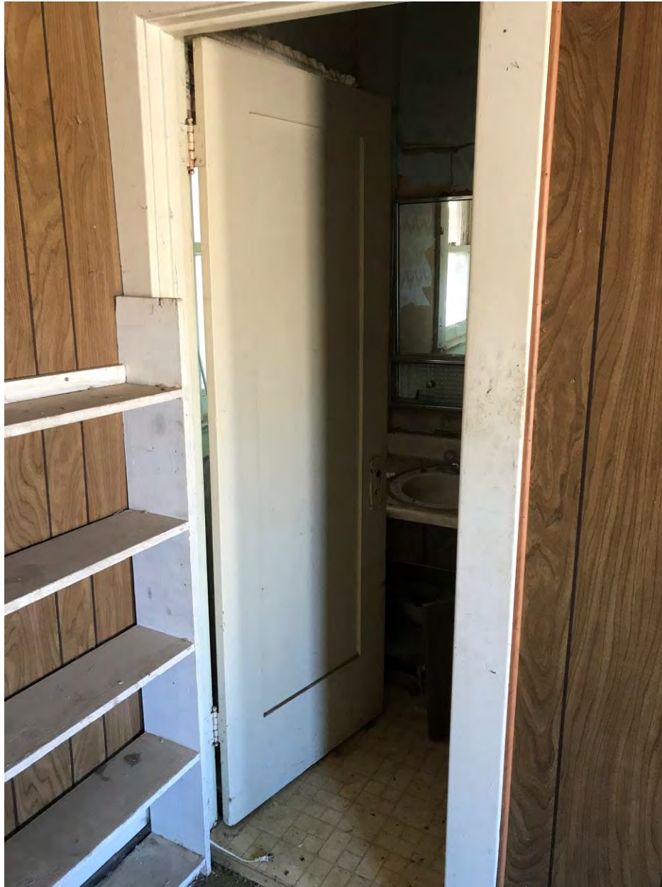
Photo 14 – Photo of vinyl sheet flooring in north restroom of building 6 that was found to contain asbestos. The black mastic behind the wood paneling located in the living room was also found to contain asbestos. Photo not included of the vinyl sheet flooring in the north entry that had asbestos containing black mastic below it.
