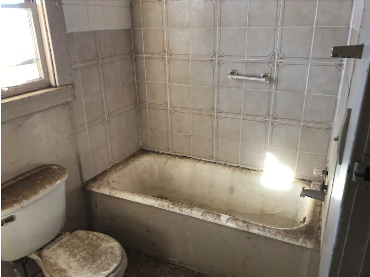
Photo 13 – Photo of porcelain tub and ceramic wall tile around tub on side D, and windows, window frames and window sills on side C of southeast restroom in building 6 that were found to contain elevated lead levels.
