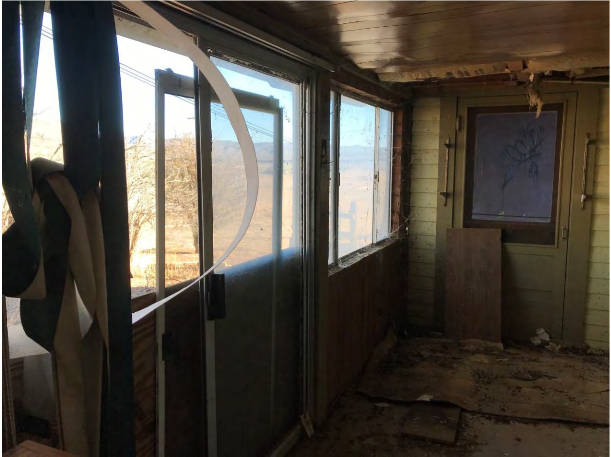
Photo 12 – Photo of posts on side B, and wood siding, door, and door frame on side C of porch in building 6 that were found to contain elevated lead levels.
