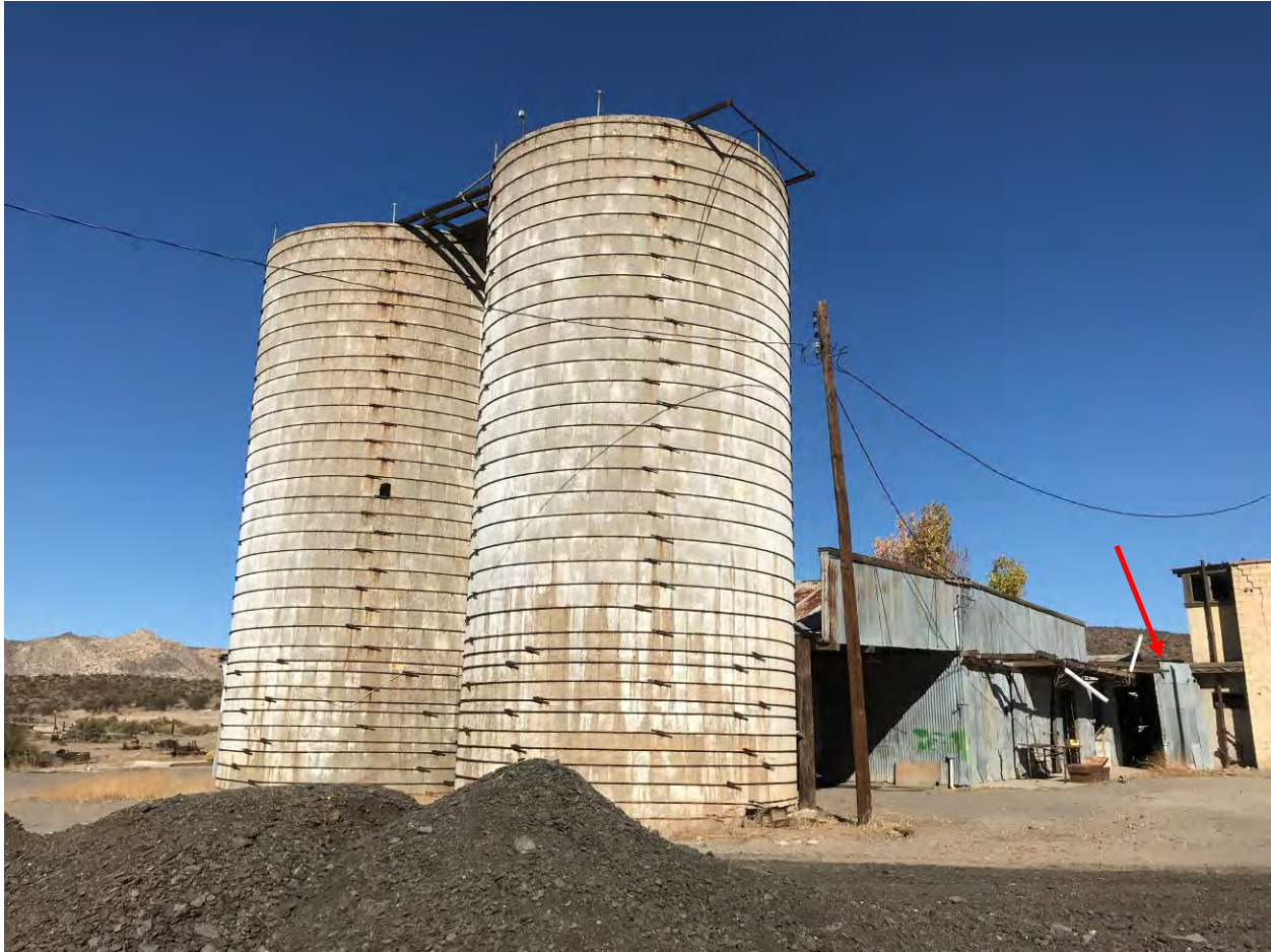
Photo 21 – Ground level view of the south side of Building 4D and the north and south silos that are on the west end of 4D. The red arrow points to the location of the layered roofing material on room 6 of building 4D that was found to contain asbestos.
