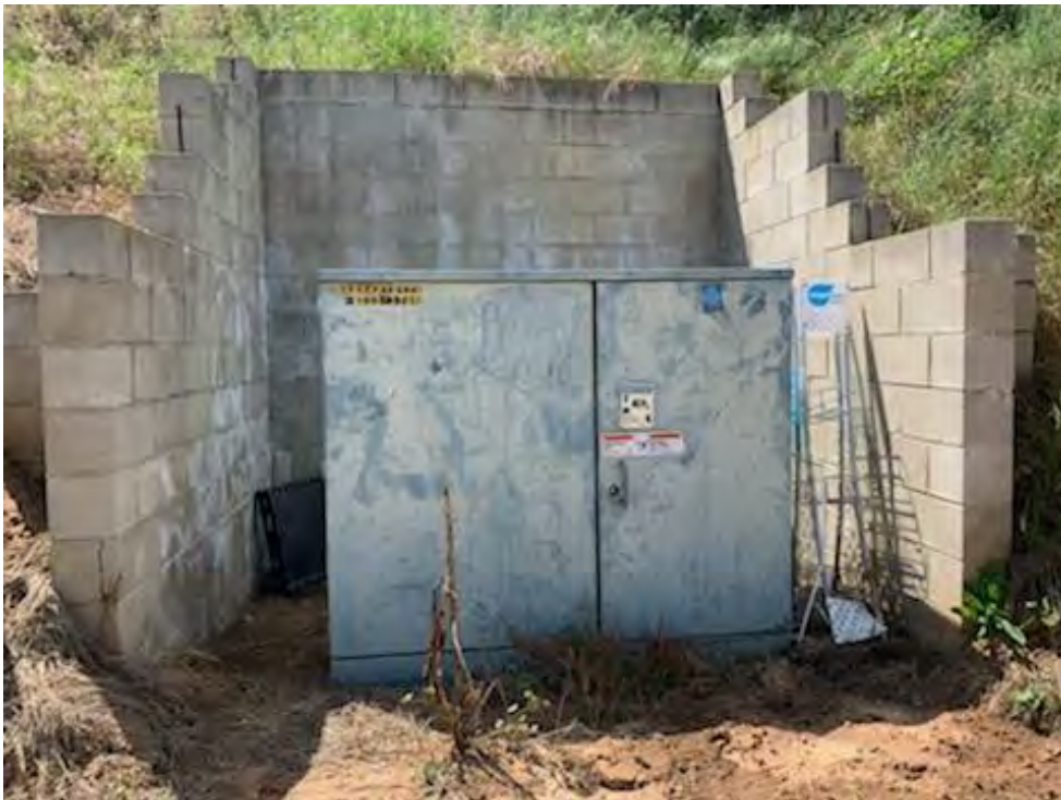
12. View west from northwest portion of property. Showing electrical cabinet and retaining wall.
