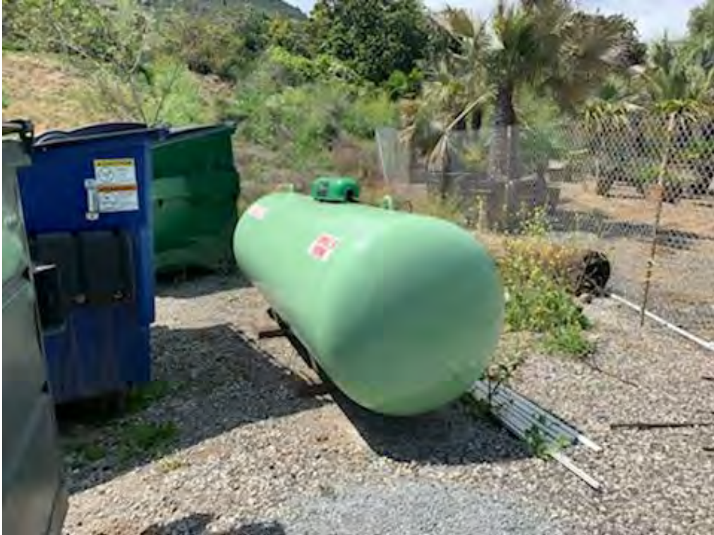
13. View northwest from northwest portion of property. Showing propane AST
