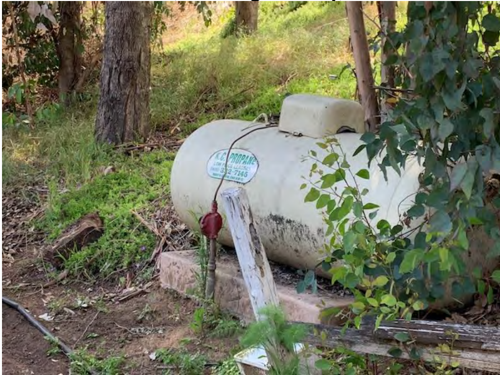
9. View southwest from west-central portion of property. Showing propane gas AST.
