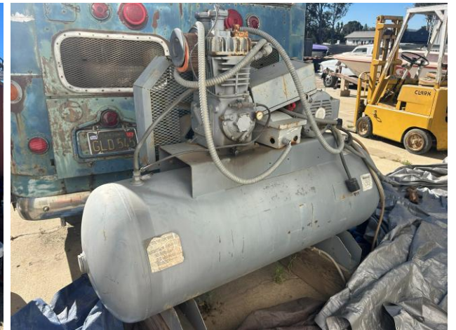
18. View of an air compressor at the former auto repair area.
