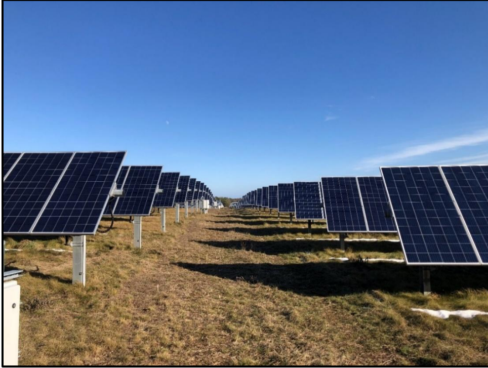
Figure 1-11. Solar Modules and Support Structures
