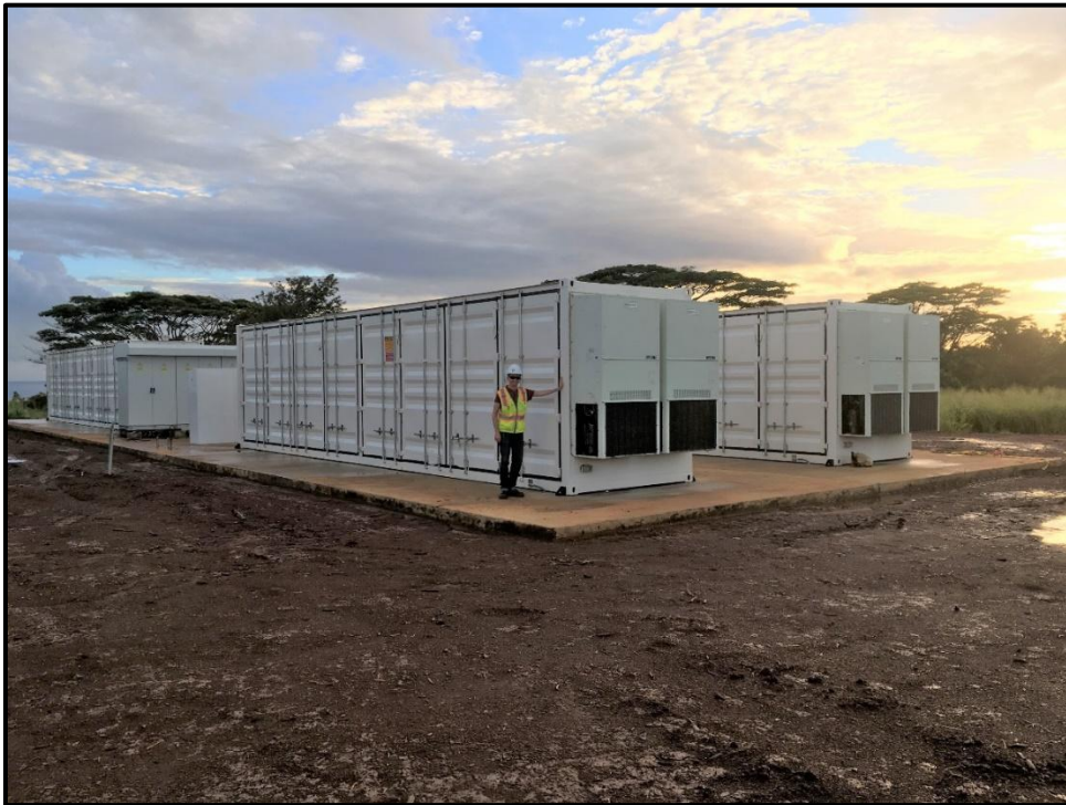
Figure 1-12. Battery Storage Container
