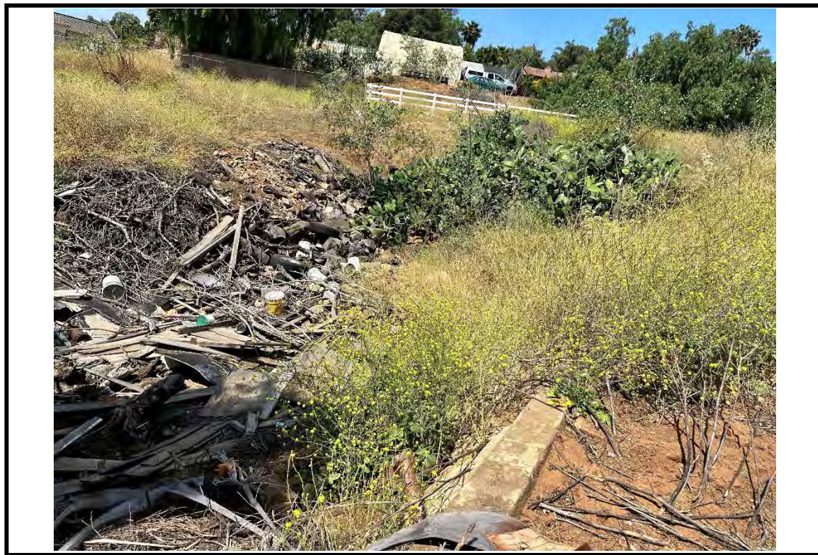
Photo Point 8. Photo of the old irrigation pond or similar. Exposed concrete is damaged. Area full of debris and no evidence of ponding. Taken on June 7, 2024 and directed west.
