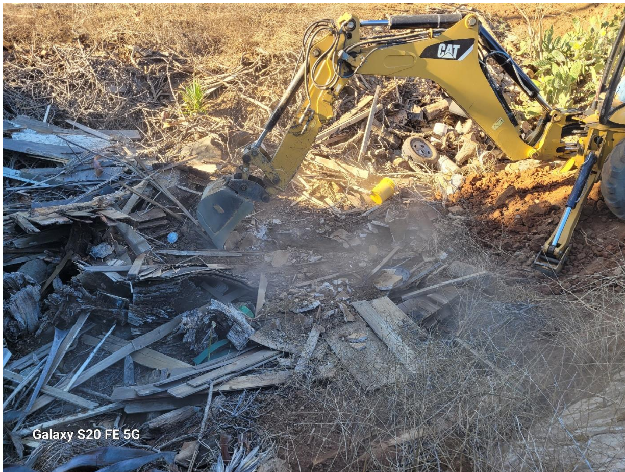
Photograph 25: Detail view of excavation performed in bottom of old pond. No additional containers were found in debris, no indication of leaking containers was found.
