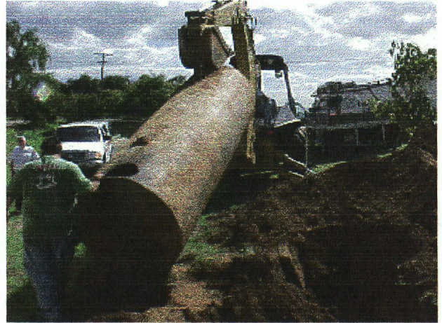
SW steel tank, very good condn.
