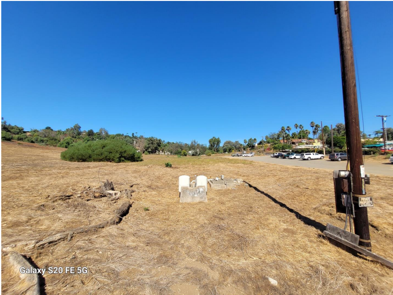
Photograph 48: View of water supply well and pressure tanks near Idaho Avenue eastern corner of site looking northwest.
