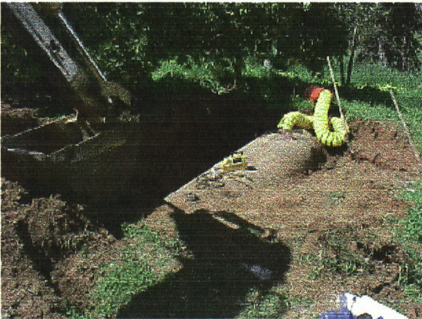
↑ (looking NW) overview during cleaning prior to pull. (note shallow depth of tank.)
