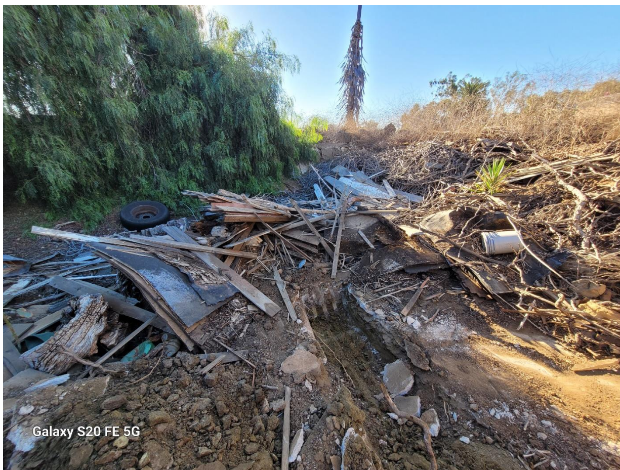
Photograph 26: Detail view of excavation performed in bottom of old pond. No indication of leaking containers was found. Bottom of pond had a concrete liner; hard native soil was encountered below liner.
