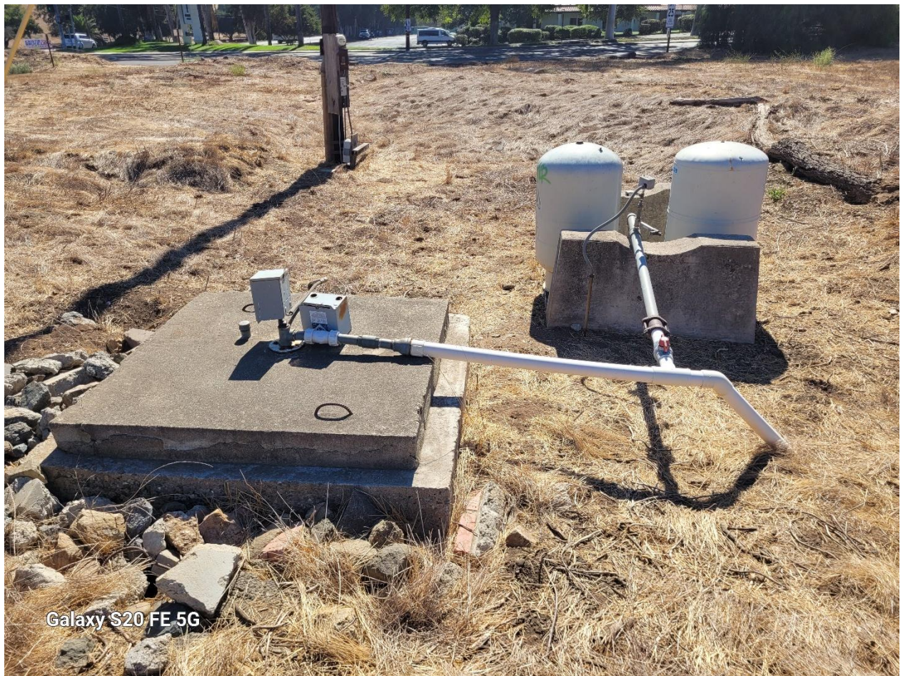
Photograph 49: View of water supply well under concrete lid, two pressure tanks and water supply piping.
