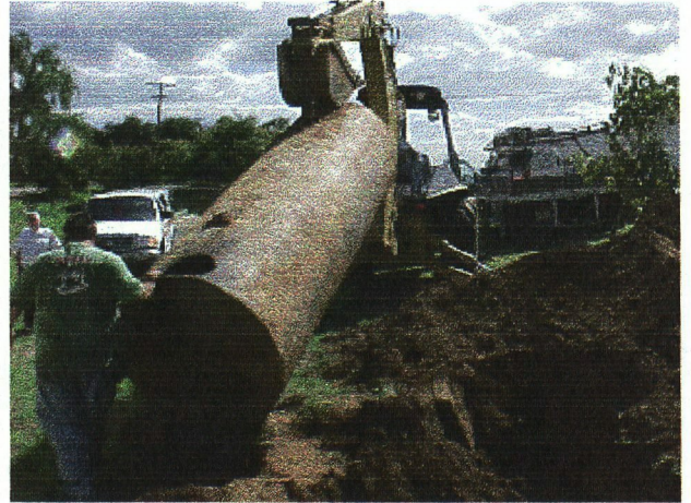
SW steel tank, very good condn.
