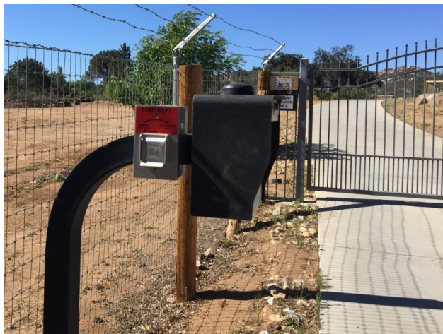
Typical Gate Override-Opening System Installation
