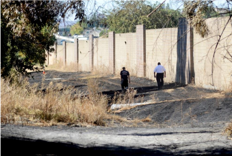
CMU Block Walls Used as Fire Barrier for Residential Sub-Division (NOTE – Extreme Mitigation Configuration)
