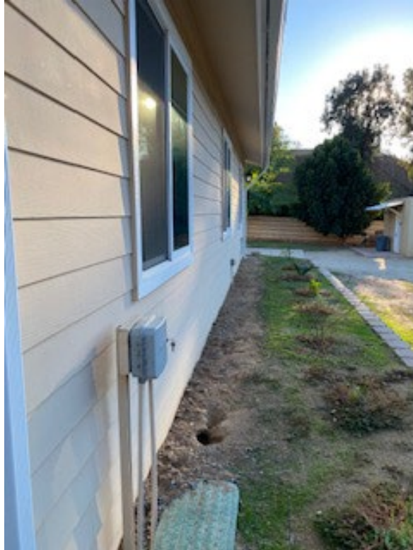
Detail of Ignition Resistant Construction Features- Hardy Board Cementitious Wall Siding; Dual-pane Windows; Enclosed Eaves
