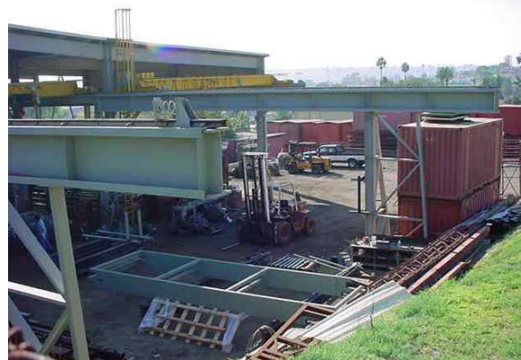
Steel fabricating plant in Spring Valley
