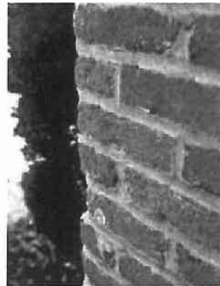
DAMAGED SANDBLASTED MASONRY
