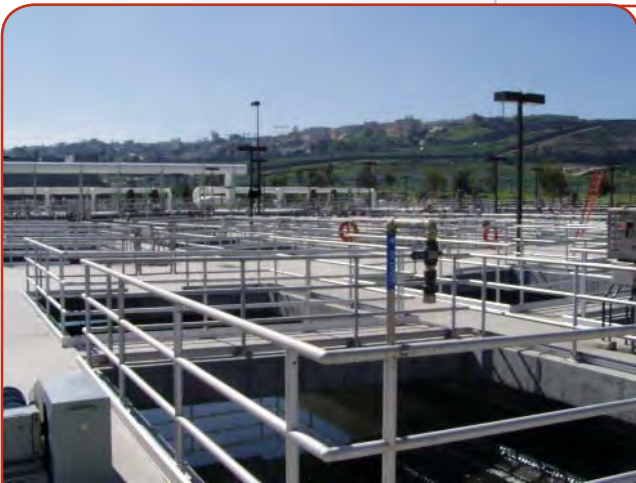
South Bay Water Reclamation Plant is one of 29 wastewater treatment and water recycling facilities in the San Diego region.
