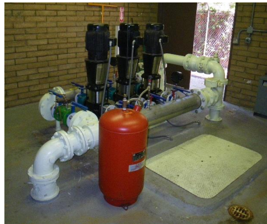
District Water Booster Pump Station (Typical)
