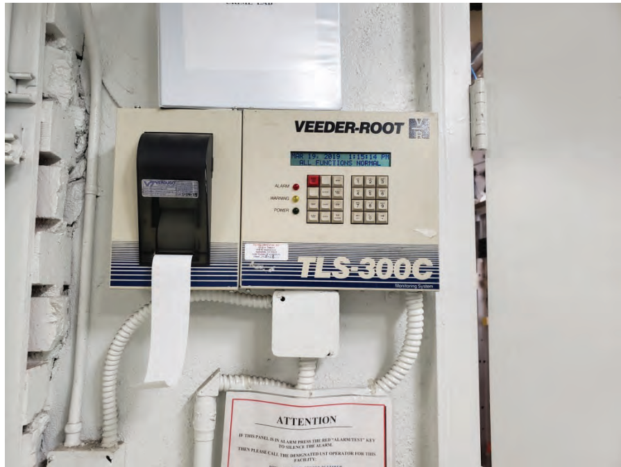
Photograph 13: View of Veeder-Root UST monitoring system.
