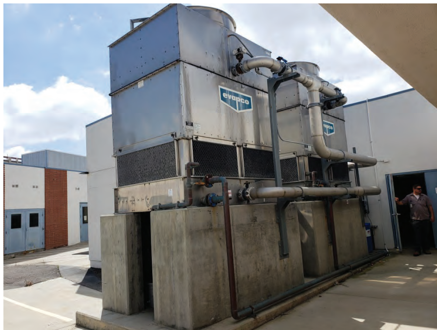
Photograph 14: View of cooling water towers, located on the south-central portion of the site.
