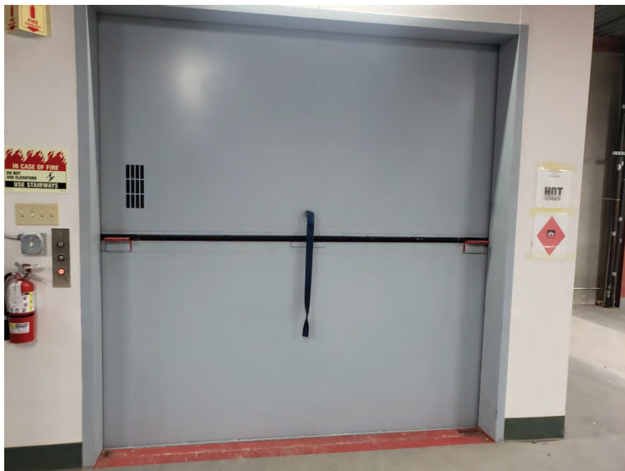
Photograph 8: View of freight elevator within the warehouse.
