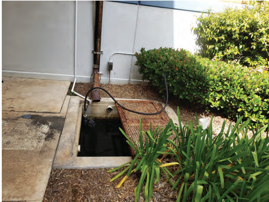
Photograph 3: View of sump and pump, located in landscaped area near the main entrance.
