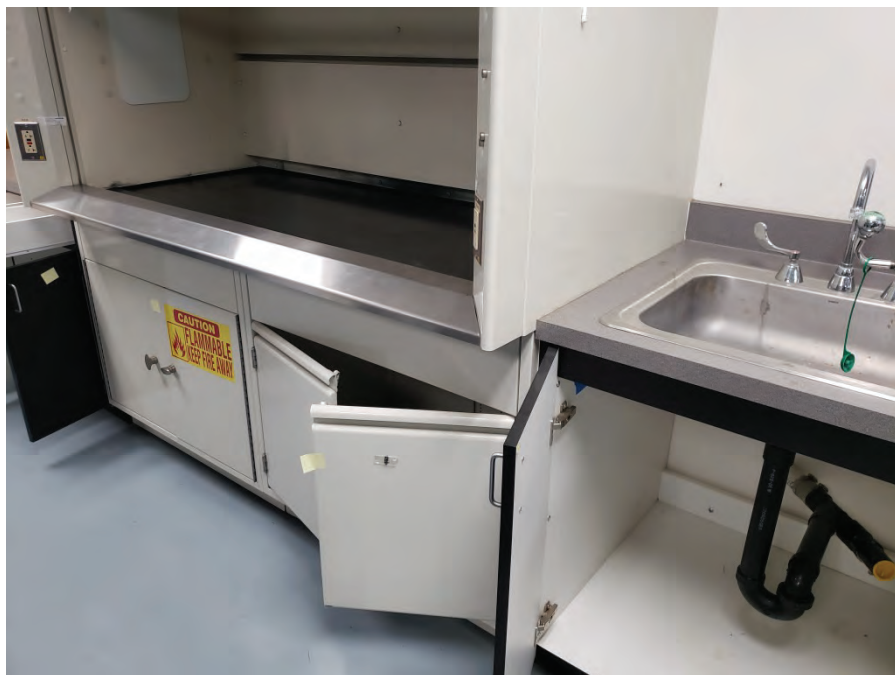
Photograph 30: View of fume hood.
