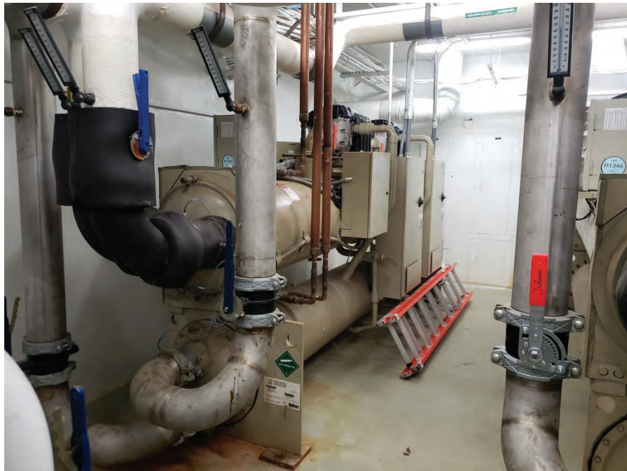
Photograph 16: View of chiller units.
