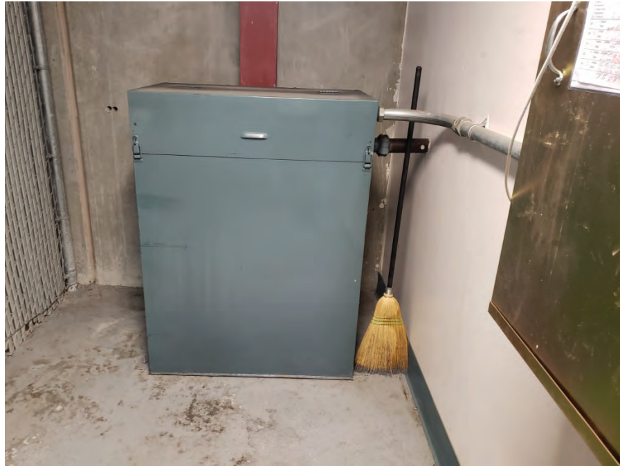
Photograph 9: View of freight elevator hydraulic fluid reservoir and pump.
