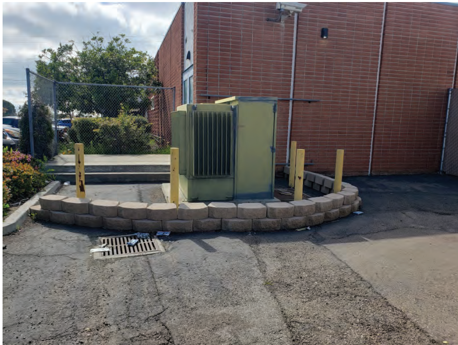
Photograph 32: View of a pad-mounted transformer and storm drain inlet, located at the south-central portion of the site.
