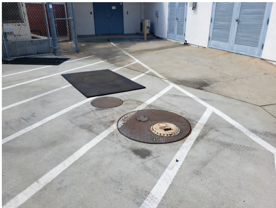
Photograph 12: View of UST access covers located to the east of the generator.
