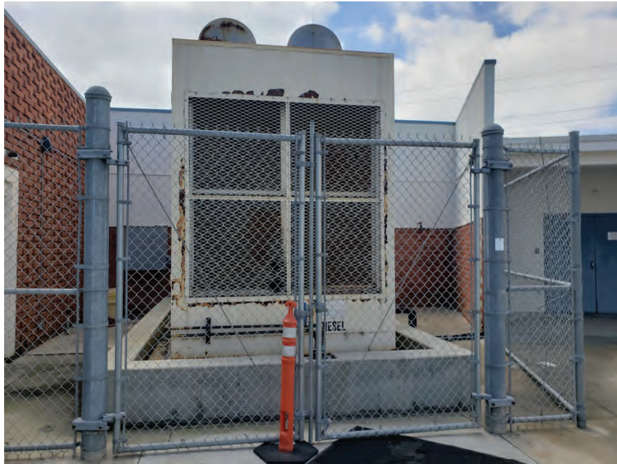
Photograph 11: View of backup generator.
