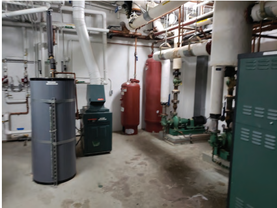
Photograph 17: View within boiler room.
