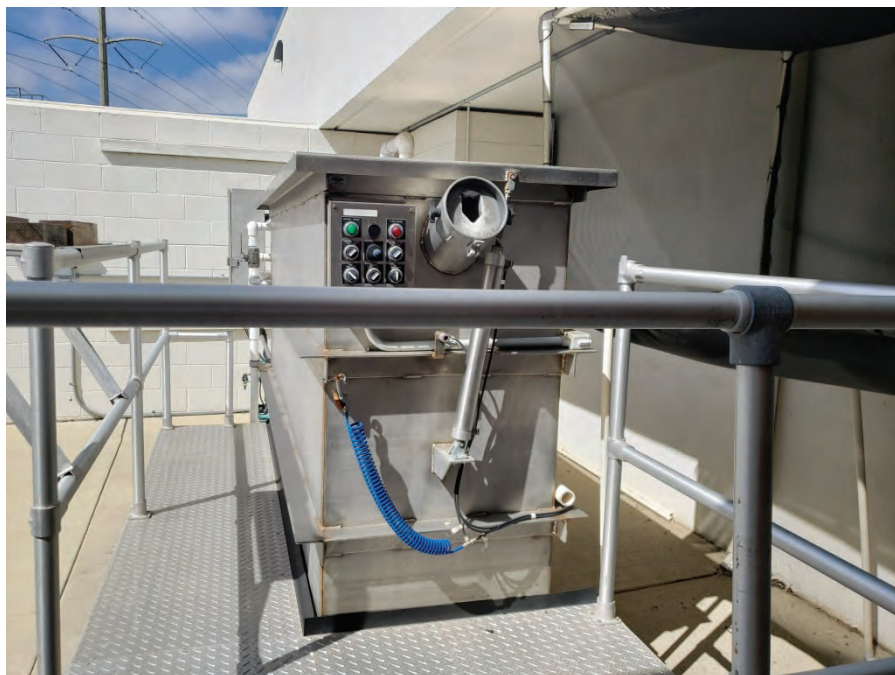
Photograph 20: View of bullet trap, located on the south eastern portion of the site.
