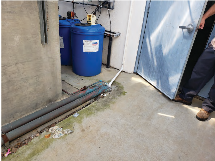
Photograph 15: View of cooling water tower treatment chemicals.
